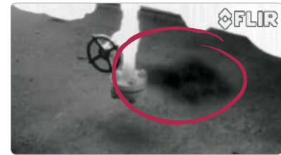
Captured gas leak from production site.
