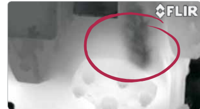
Captured gas leak.
